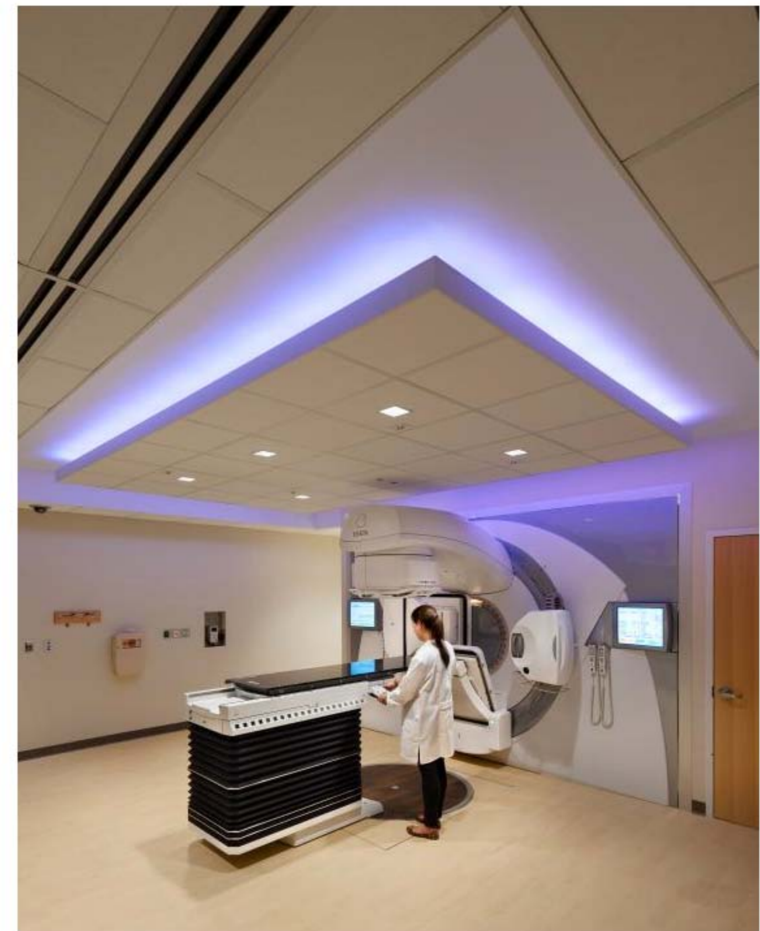
The cancer center houses two concrete linear accelerator vaults on the first floor, which support the radiation oncology program. Color-changing LEDs create a soothing environment for patients as they receive treatment. Light-colored, wood-look flooring contrasts with dark-colored, wood-look millwork to finish the interior. Decorative sliding acrylic panels conceal treatment accessories from patient view. Photo: ©Chris Cooper Image 5 of 5
